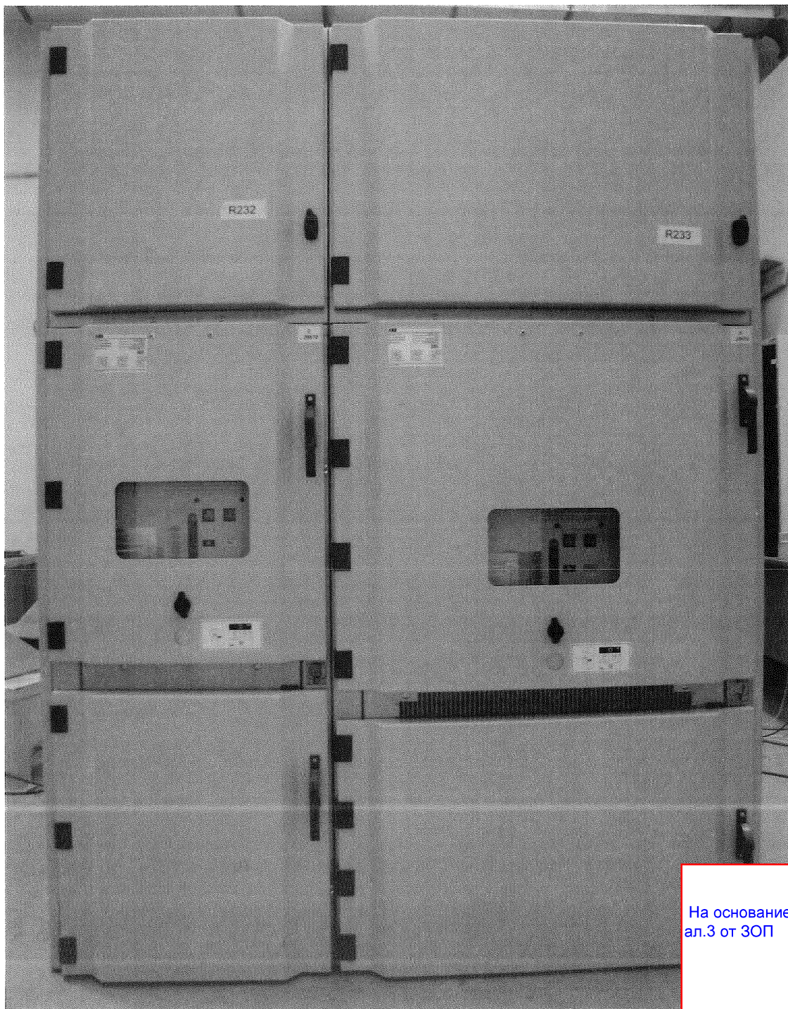
Photo 1: Front view of switchgears
